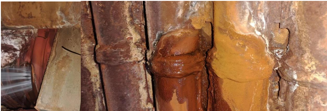
图3-4 振动造成水冷壁鳍片撕裂
