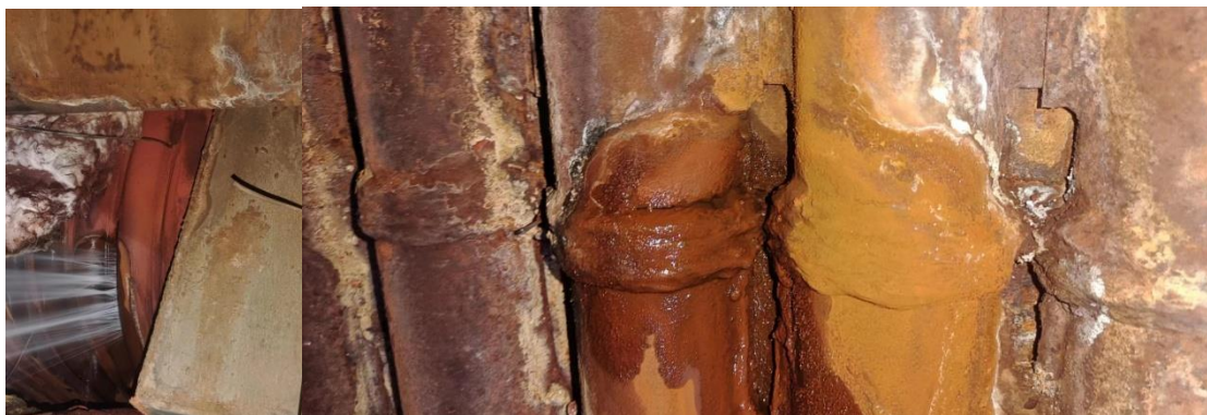
图3-4 振动造成水冷壁鳍片撕裂
